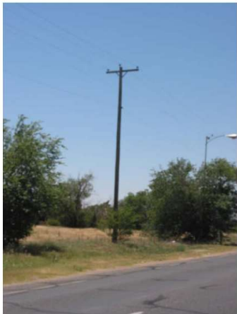
ETL: Single Wood Pole
