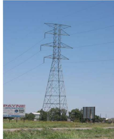
ETL: Metal Truss Tower (WSEC 2006)
