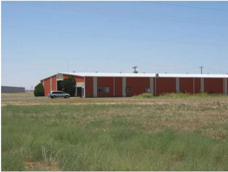
MBS: Metal roof and wall panels; gable roof shape; Z or C-shaped purlins and girts; single-bay rigid frames; x-bracing parallel to ridge
