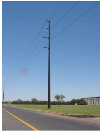
ETL: Single Steel Pole
